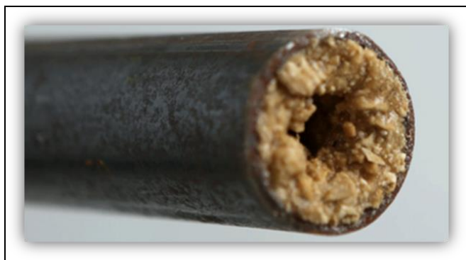
Figure (1): Calcareous scaly deposits in water distribution systems
