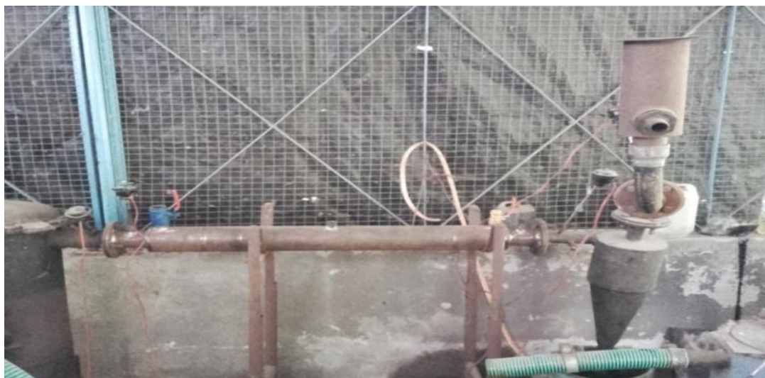
Fig. 2: Photograph of gasifier-cyclone assembly along heat exchange
