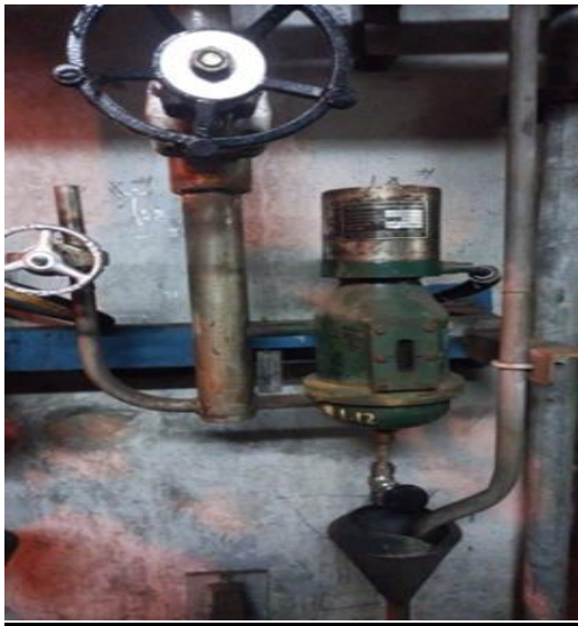
Figure 8. Leak drain sensor that broken.
