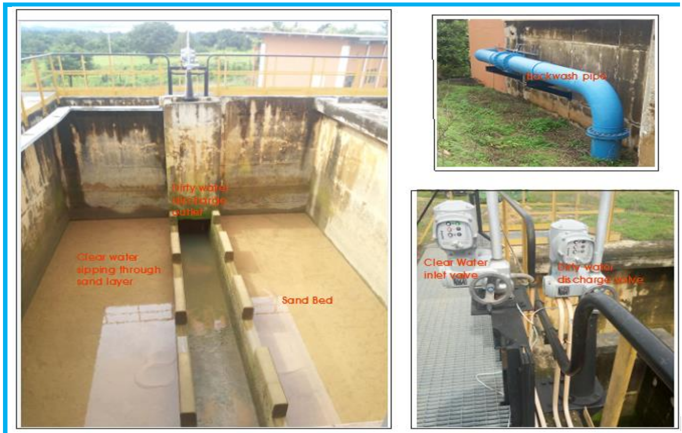
Figure 19: Rapid Sand Filter at Mada Water Works
