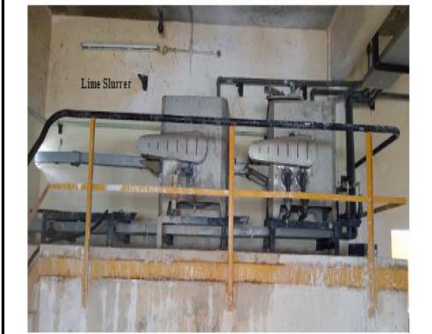
Figure 10: Lime Tanks and Lime Slurrer
