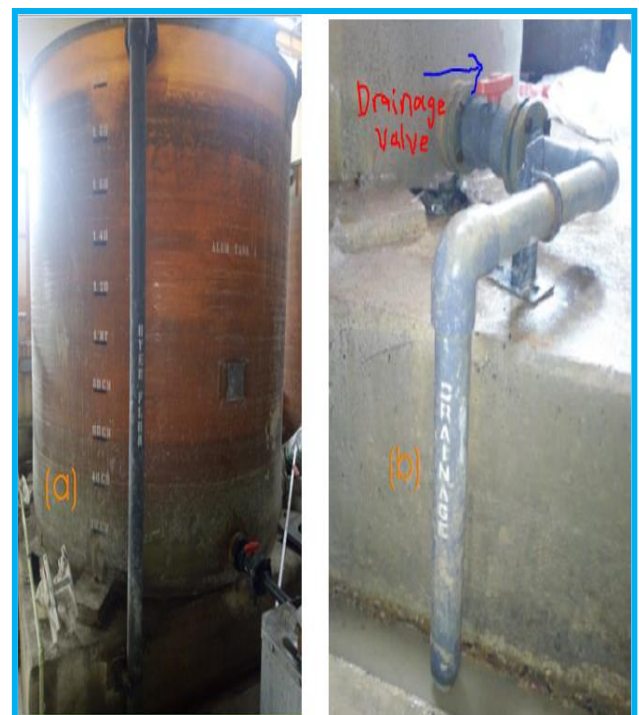
Figure 7: (a) Overflow and (b) Drainage Outlet Pipe
