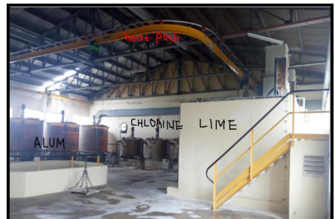
(a) Chemical Building depicting the Chemical Tanks
