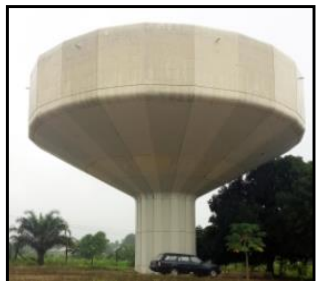
(b) Wash Water Tank
