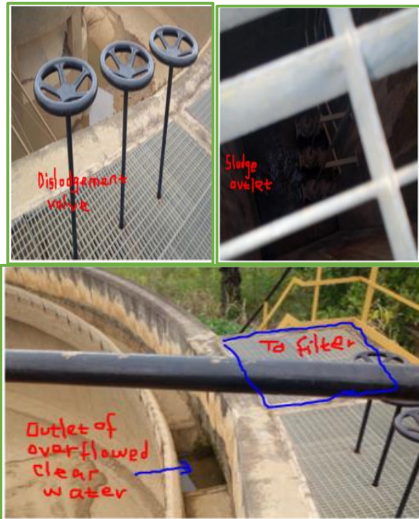
Figure 18: Dislodgement Valves and Sludge Outlet
