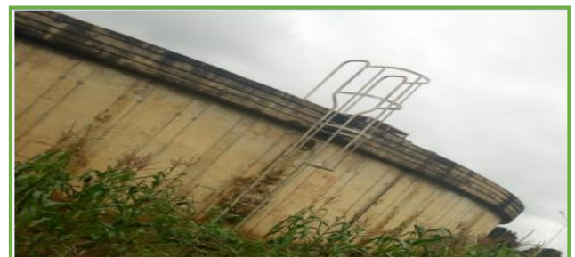
Fig. 17: Balancing or storage tank
